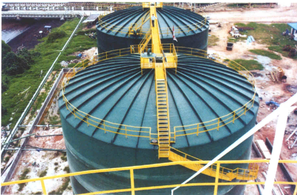
An aerial view of the two huge acid tanks.
