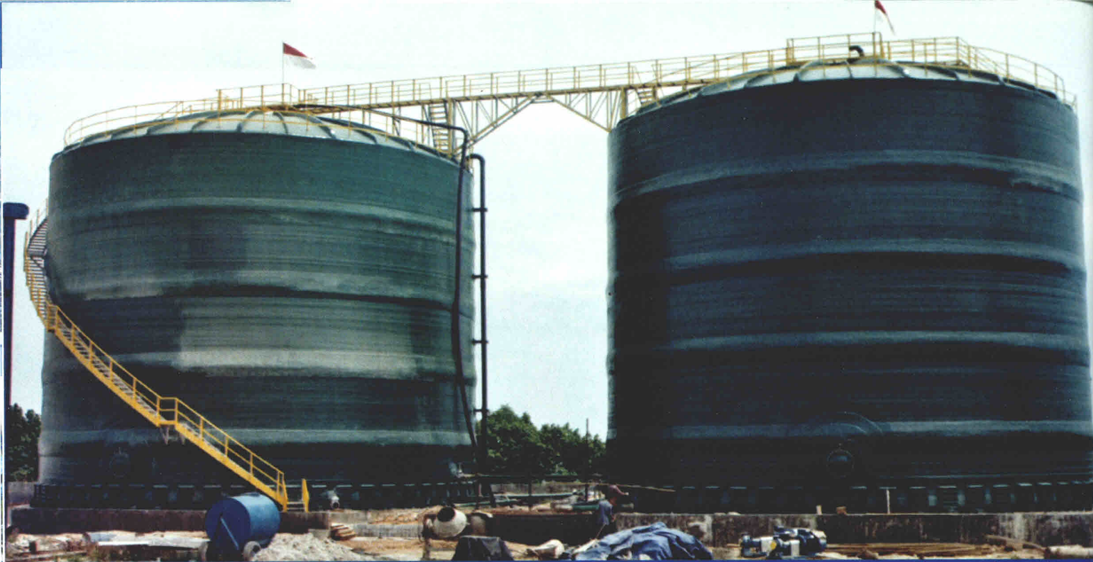
The two phosphoric acid storage tanks
